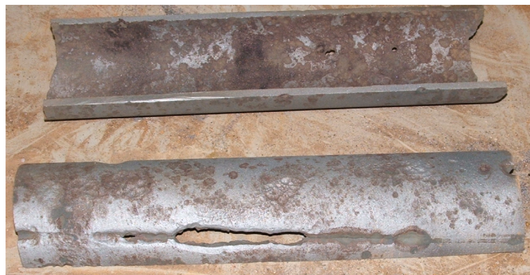
Fig. 10. Pipe blowout with the presence of longitudinal crack. Samples provided by Bristol Water, UK.
