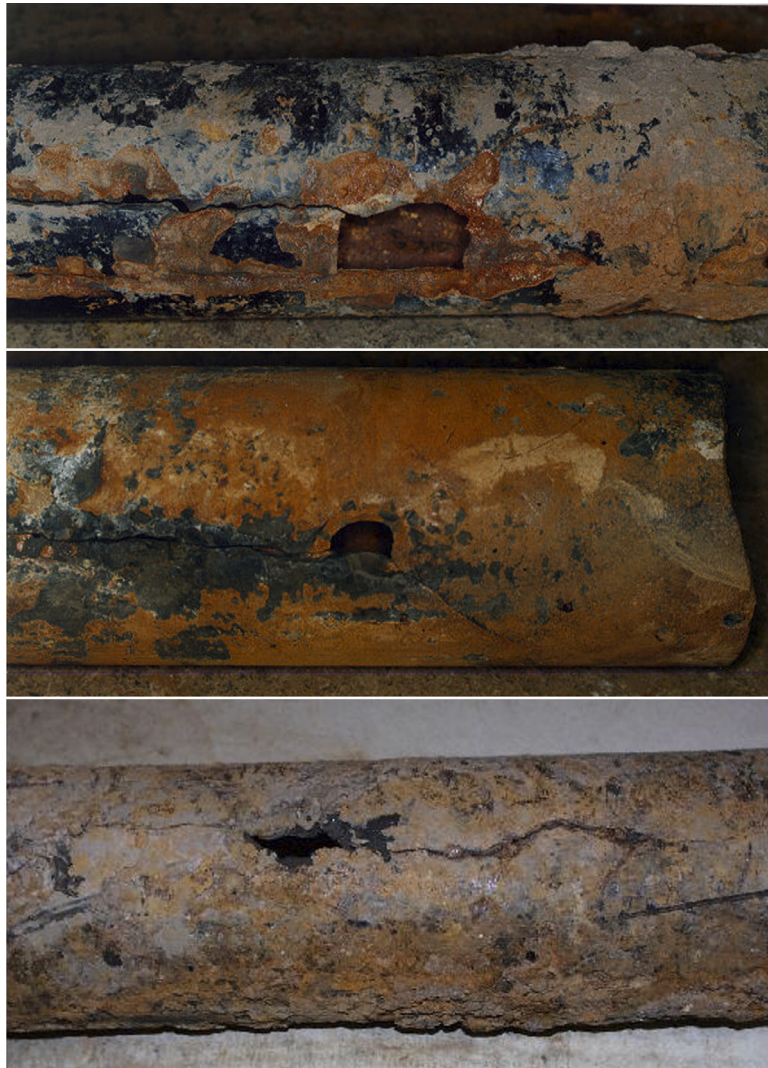
Fig. 8. Longitudinal failures in water distribution pipes due to initial corrosion pits. Samples provided by Bristol Water, UK.
