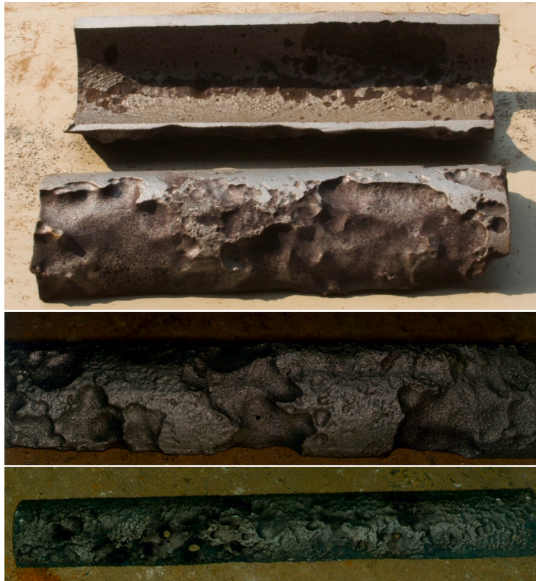
Fig. 7. Examples of pipe deterioration due to corrosion pits and patches after sandblasting pipes. Samples provided by Bristol Water, UK.
