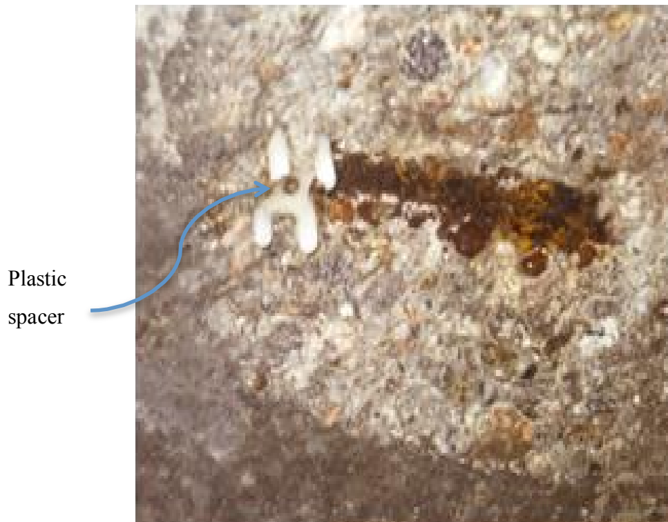
Figure 2.7 Local chloride-induced corrosion adjacent to plastic spacer location. [Rostam, 2005]
