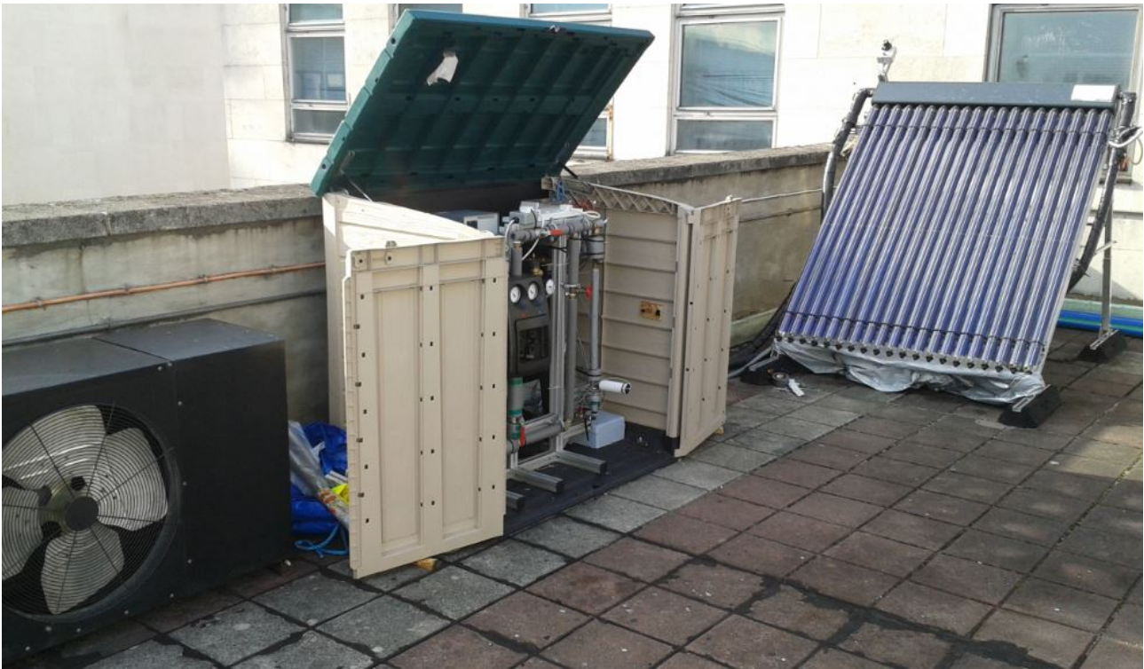
Figure 5.3: Experimental apparatus including air-cooled heat exchanger (left), solar collector array (right), and pump station (centre).
