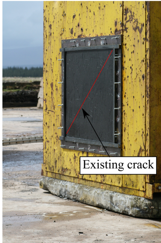
Figure 3-16: Existing diagonal crack location.
