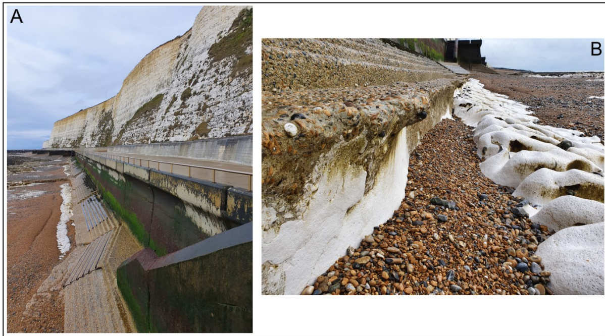
Figure 6.4. The Saltdean location. Photograph A: splash wall, undercliff walk, seawall with steps and shingle beach in front of them. Photograph B showing a part of the seawall directly on the shingle beach. The erosion at the seawall has exposed the seawall foundations and the chalk that underlies it. The bottom step has slight concave shape from nonstop wave erosion.
