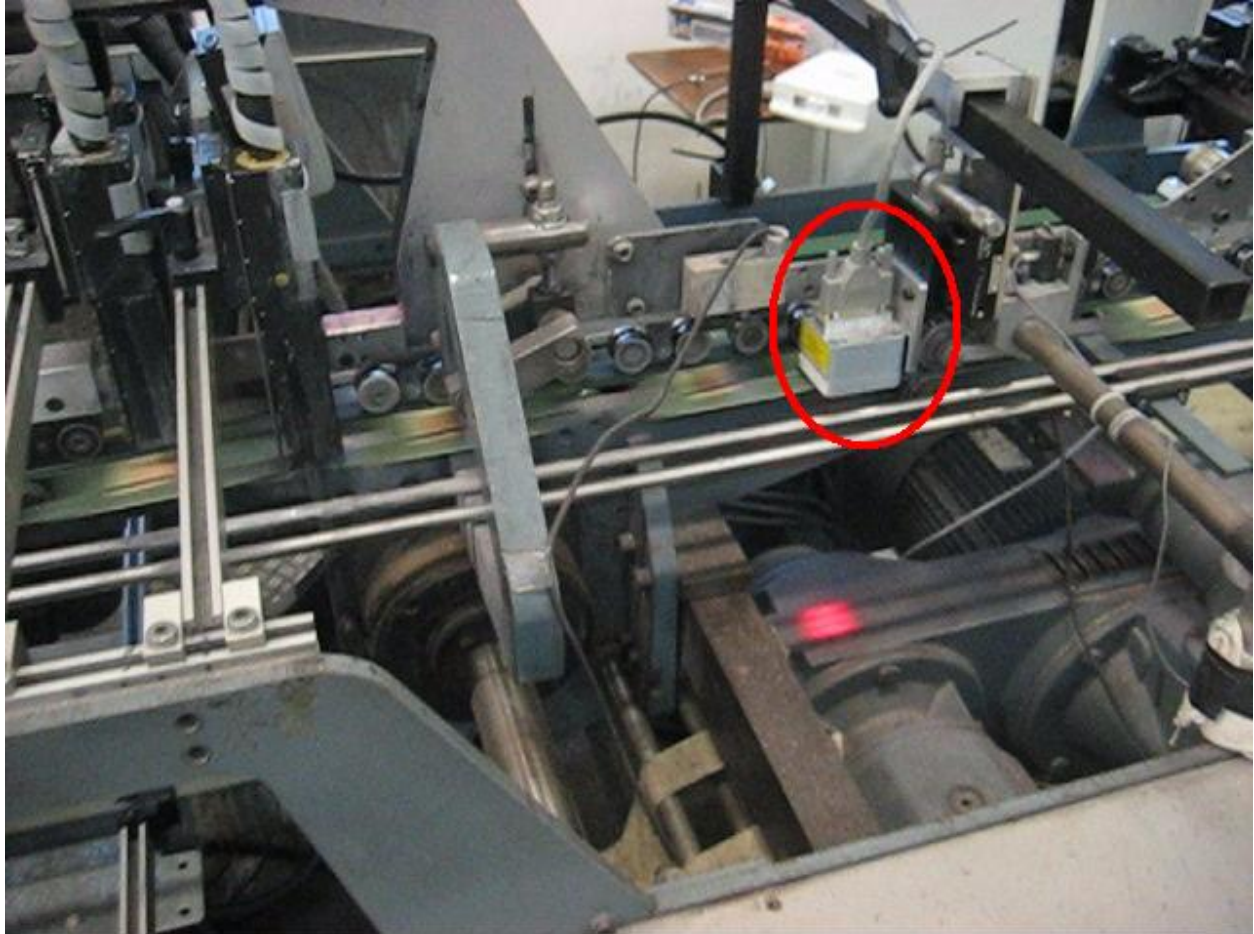
Figure 3.1 An LSA sensor head (circled) mounted above the conveyor belt on the machine which processes individual cartons, before they are formed into boxes.
