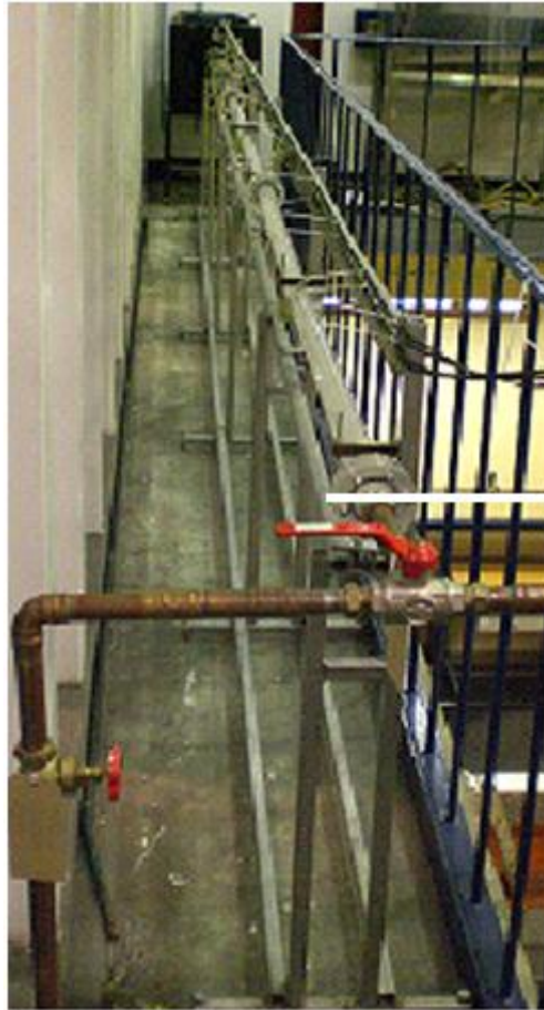
Figure 4.1. Photograph of the horizontal pipe.
