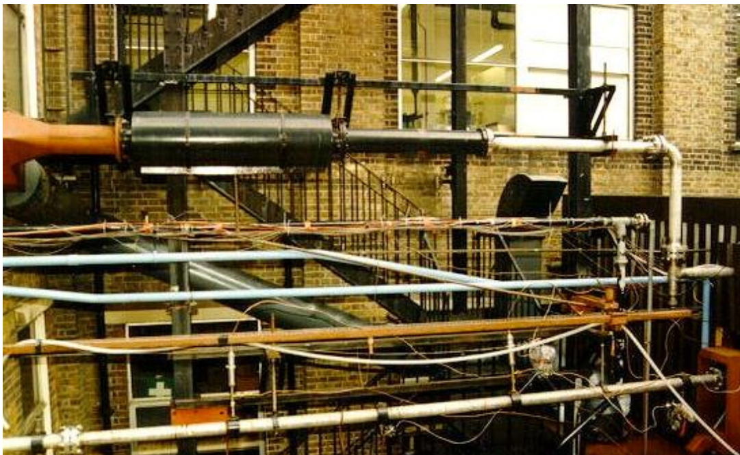
Figure 4.16. The air discharge line and silencer.
