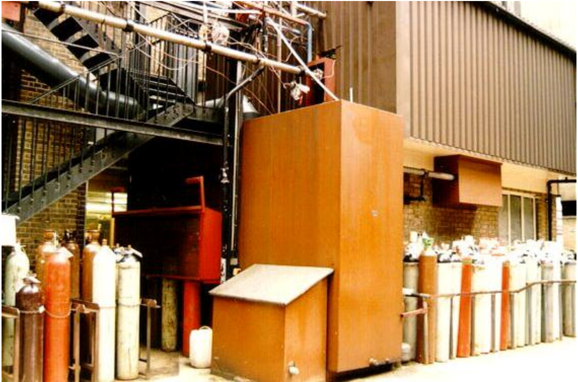
Figure 4.17. The dump tank.
