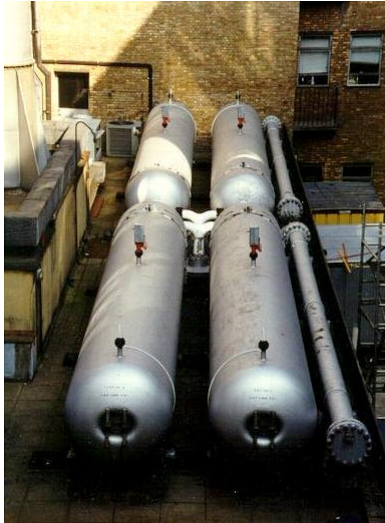
Figure 4.10. The high pressure air supply tanks.
