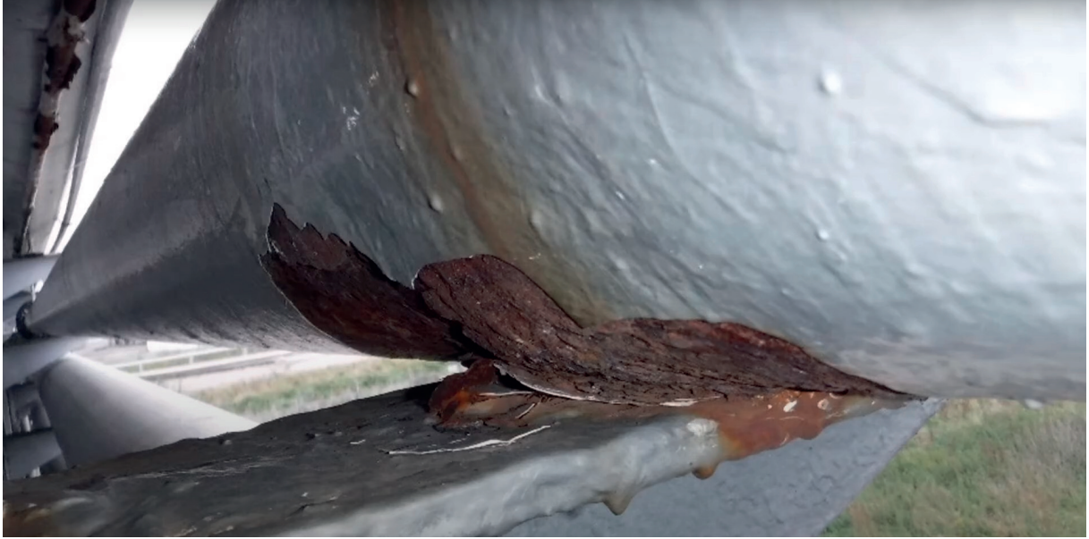
Figure 1.1: Spotlight on a corrosion patch at pipe support. In order to assess service-life, quantitative measurement of the remnant wall thickness at this point is vital. Source: Guided Ultrasonics Ltd., January 2022
