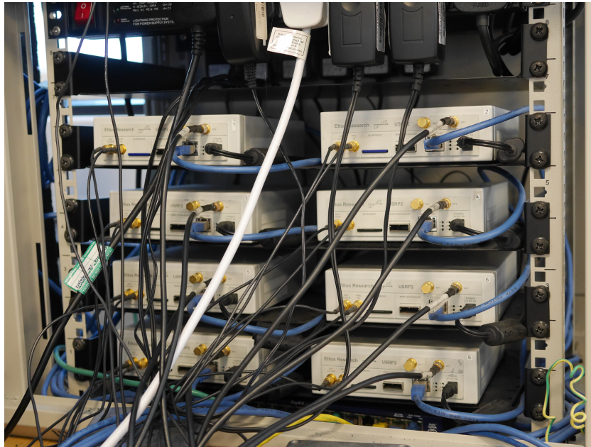
Figure 3.2: Multi-USRP hardware configuration for the 9-element array (8 out of 9 Rx USRP boards are shown here), USRP boards share a common clock that is generated by a GPS module.
