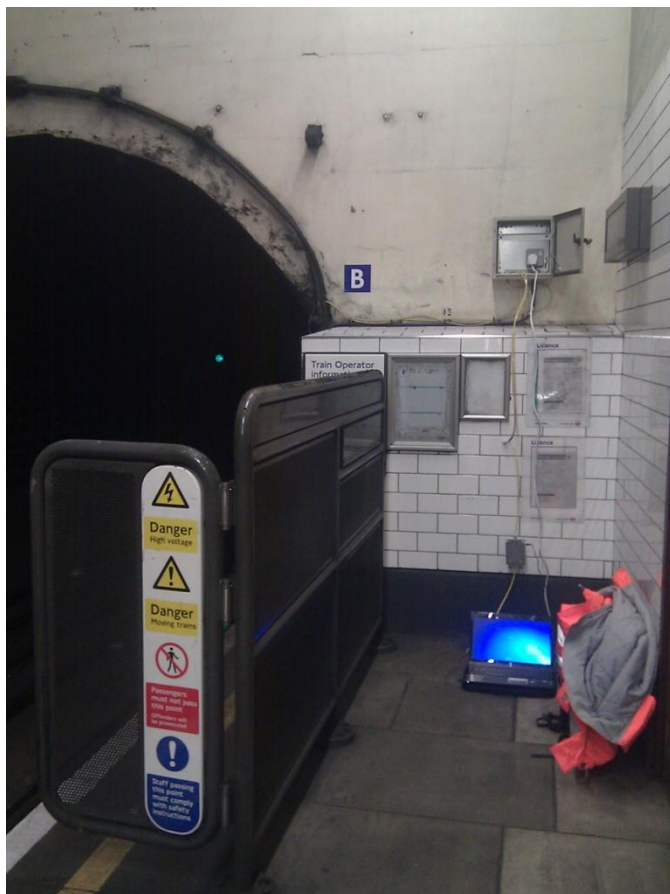
Figure 3-21. Additional datalogging unit on the eastbound platform headwall.
