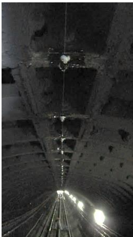
Figure 3-28. Fibre optics fixed to the key pieces along the crown of Central Line.
