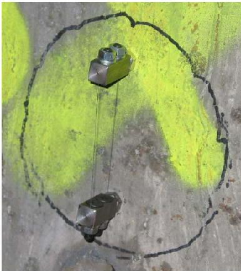
Figure A-11. Vibrating wire strain gauge installed on skin of tunnel segment (Tube Lines, 2006).
