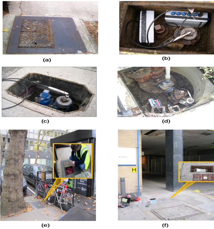
Figure 4.29. (a) An outside view of a fire hydrant with a metal cover, (b)-(d) inside view of typical fire hydrants with monitoring equipments. (e-f) deployment sites for conducting field-trials, referred to as FH1 and FH2 respectively. Photographs are courtesy of Dr. Ivan Stoianov and Asher Hoskins from Civil Engineering Department at Imperial College London.
