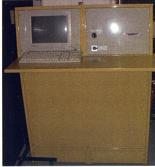
Figure 5.7 Engine control panel
