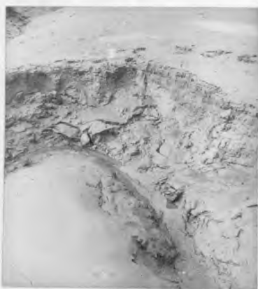
PLATE 63. ROTATIONAL SLIPS IN SIDE OF CREEK CHANNEL.
