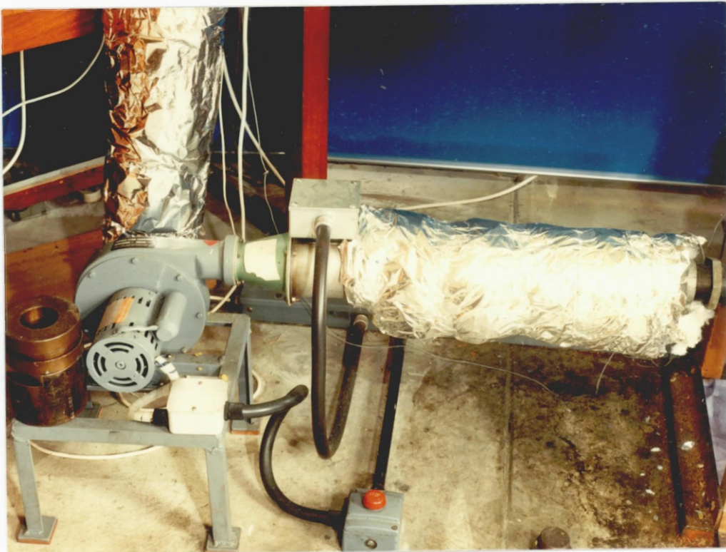
Figure 4.6 The heating system
