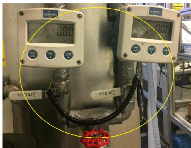
Figure 4.6: Flow meter positioned closely to the elbow.
