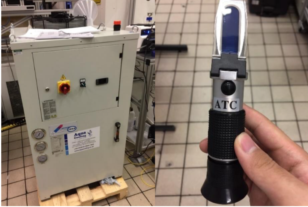
(a) Aqua cooling chiller.
