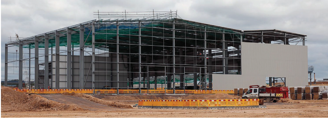
Figure 1.2: HS2 precast manufacturing facilities constructed as a multi-span steel portal frame (NSC, 2021)
