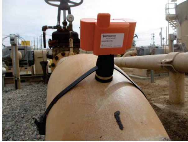
Figure 1.1: ET210 EMAT-based monitoring system (Permasense Ltd., Horsham, UK, an Emerson company, US). Image from http://www.permasense.com/technology.php (Oct. 2016).
