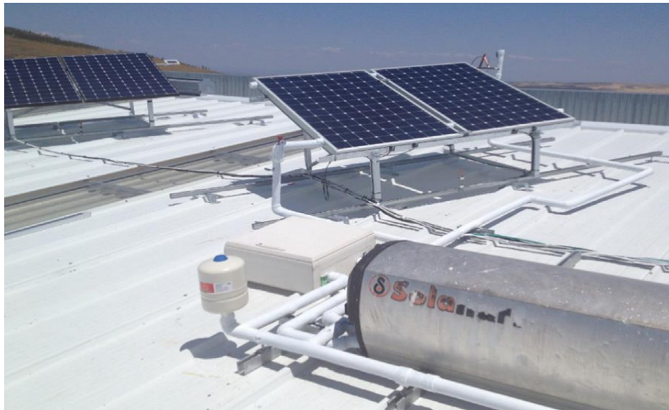
Fig. 24. Photograph of solar water heating system with PV-T collectors [181].
