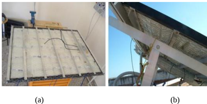
Fig. 18. (a) PCM encapsulated in plastic bags, and (b) PV-PCM integrated panel [134].
