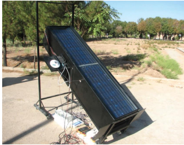
Fig. 8. Photograph of the practical implementation of the PV-T air system used in Ref. [74].
