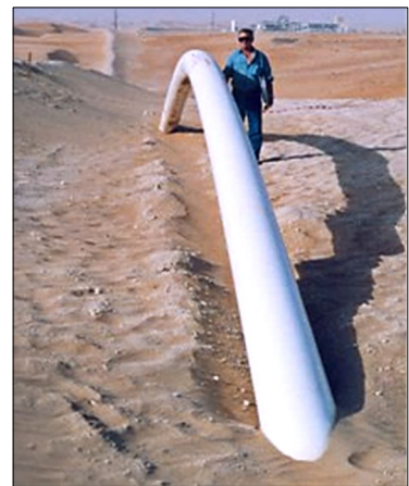
Figure 2.6 Upheaval buckling of a pipe
