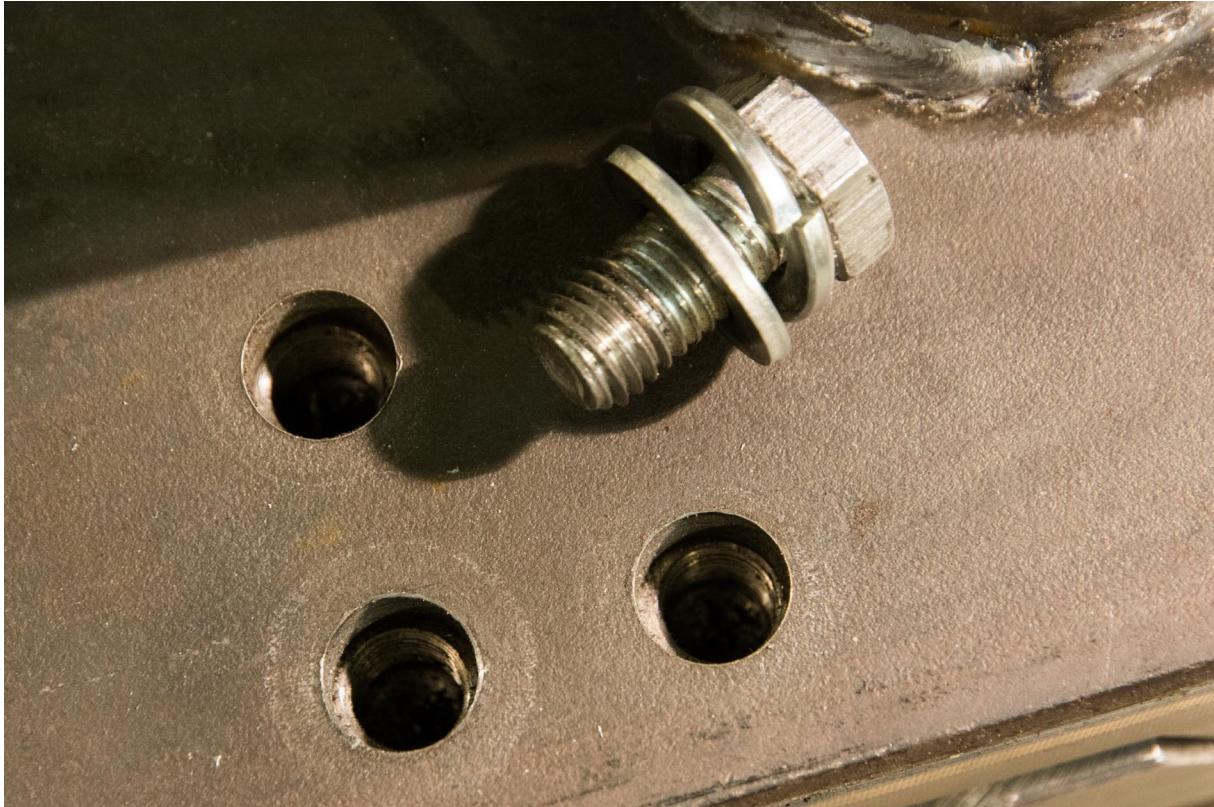
Figure 4.7: Oversized bolt holes in an end plate at UPC.
