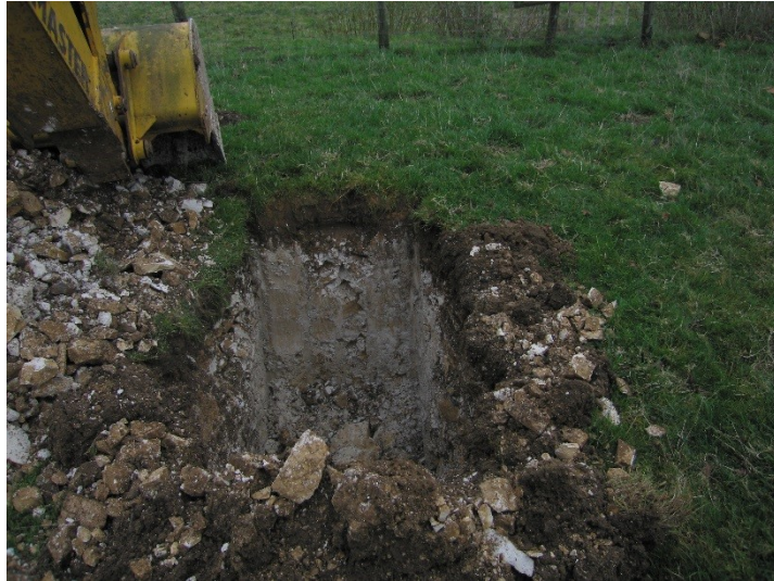
Figure 3-9: Image of the installation of Station ELSH (Baptie 2015). The thin topsoil can be seen with the typical white of the chalk beneath. However, the station foundations are clearly below the topsoil. The chalk appears rubbly and poor quality and was described as white and clayey (Laughlin 2014).
