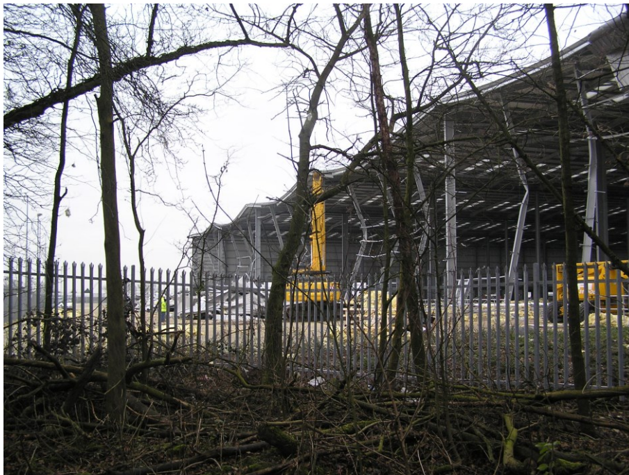
Figure 1-1 – Image of damage to warehouse at Buncefield (Author's photograph)
