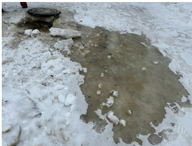
Figure 4.4: Sewage overflow incident from a septic tank (February 2024).
