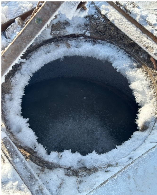
Figure 4.2: Crust formed inside the septic tank.
