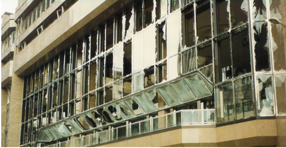
Figure 1.1: Failure of a building facade subject to blast loading (courtesy of David Smith at Arup).
