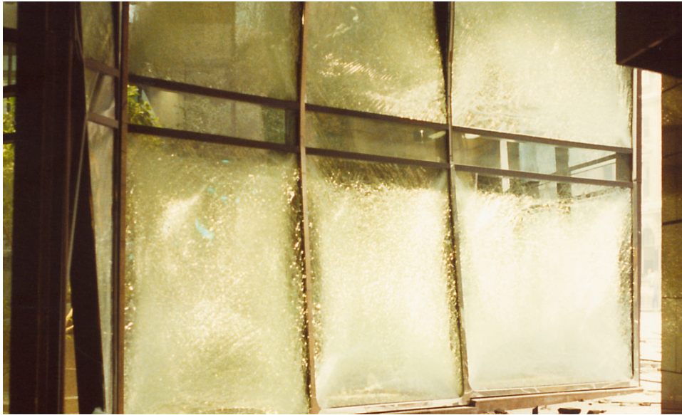
Figure 1.2: Cracked laminated glass following a blast explosion (courtesy of David Smith at Arup).
