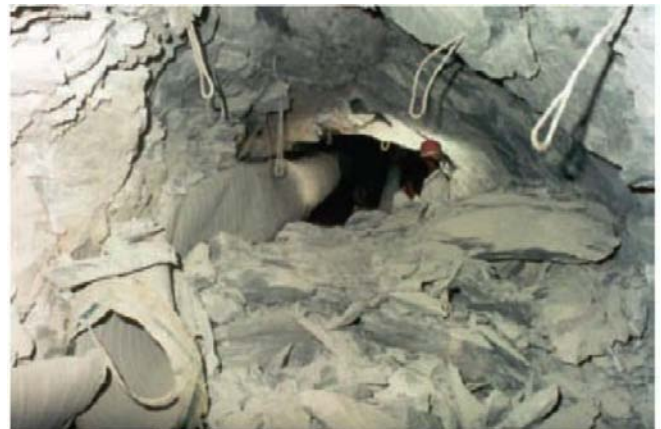
Figure 1. Rock burst damage and fragmentation.
