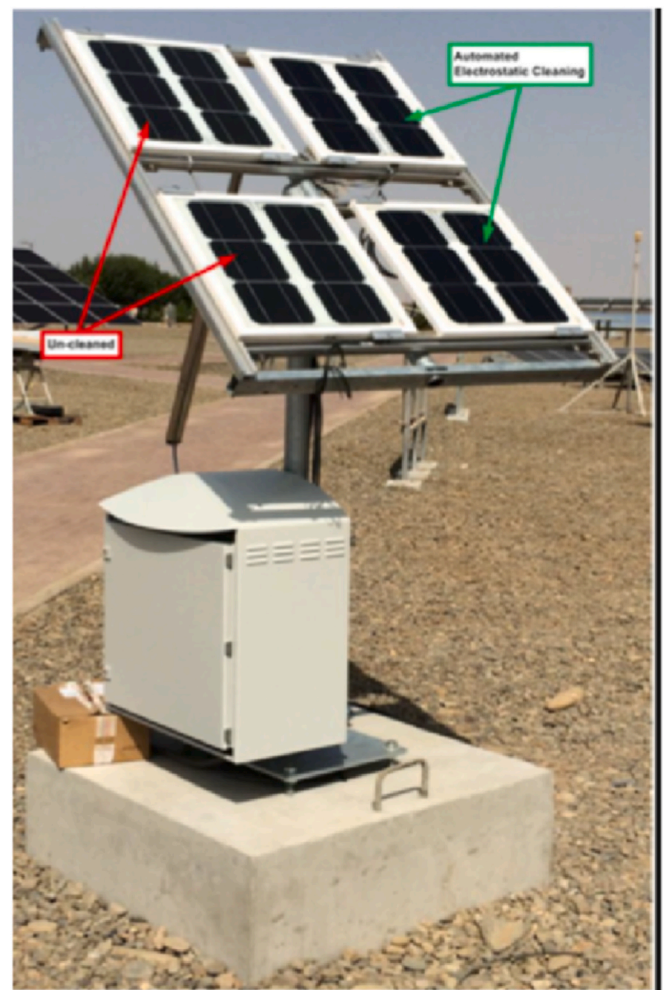
Fig. 10. Field test of EDS system in Saudi Arabia [25].
