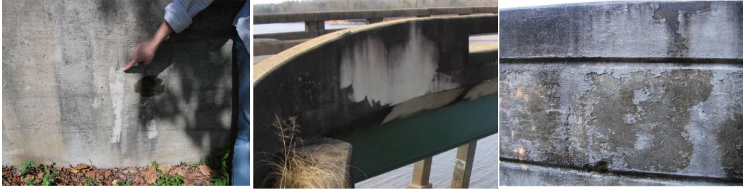
Figure 1. Surfaces of concrete structures covered and affected by biofilm where several fungal species, including Cladosporium and Aspergillus , have been isolated [2]
