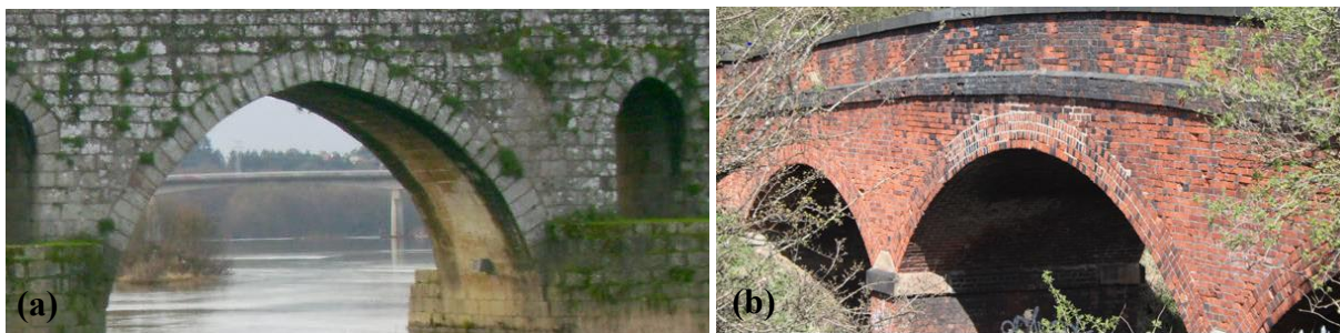
Figure 1: (a) Roman stone-bridge over the Limia river (Portugal) and (b) Brick Rail bridge, Stapleford (UK).
