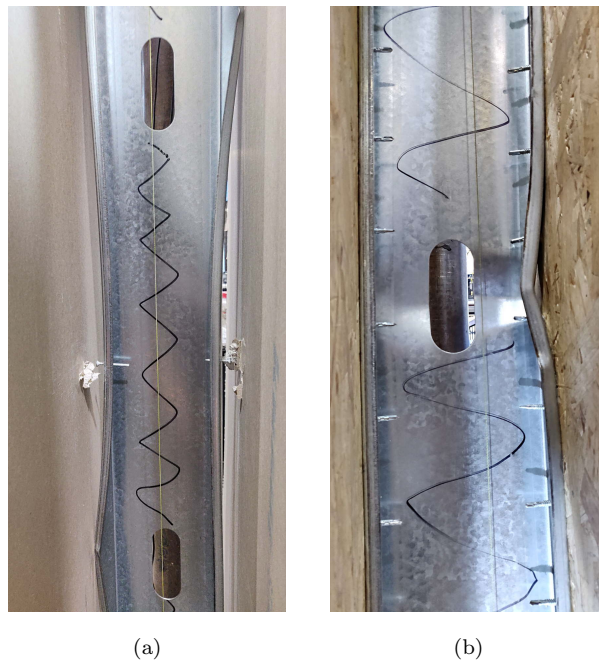
Figure 19: Typical failure modes: (a) distortional buckling (and pull-through failure of connectors) for a member under compression and (b) local buckling at a service hole for a member under bending
