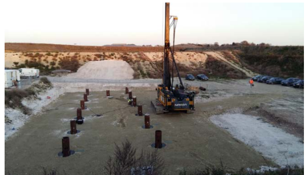
Figure 14 Piling operations underway at St Nicholas at Wade for ALPACA JIP programme; November 2017.
