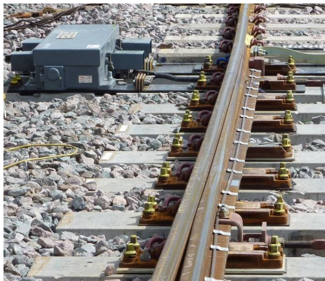
Figure 2-1: Picture of a 'half set' of switches, showing the variation profile longitudinally for the switch rail and the contact conditions (light sections on the head of the rail)
