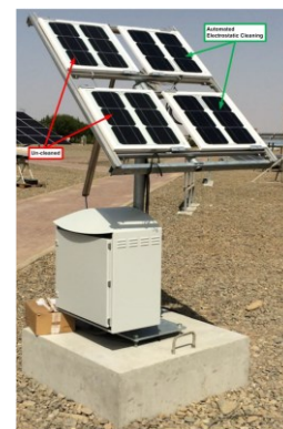
Fig. 2.10 Field test of EDS system from CleanFIZZ at KAUST near Jeddah in Saudi Arabia [62].
