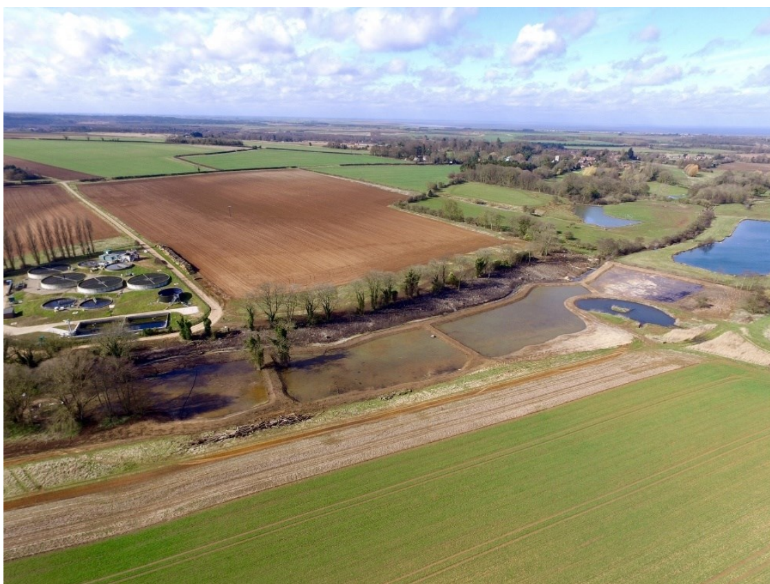
Figure 7.2 The area by the Ingoldisthorpe Recycling Centre after the completion of the works. Credit: William Morfoot
